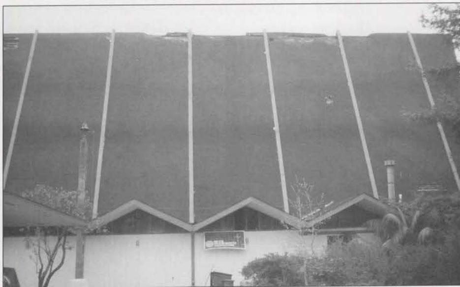
Trinity Presbyterian Church roof line where flames broke through. Tons of water went through, collapsing the organ chamber ceiling below.
