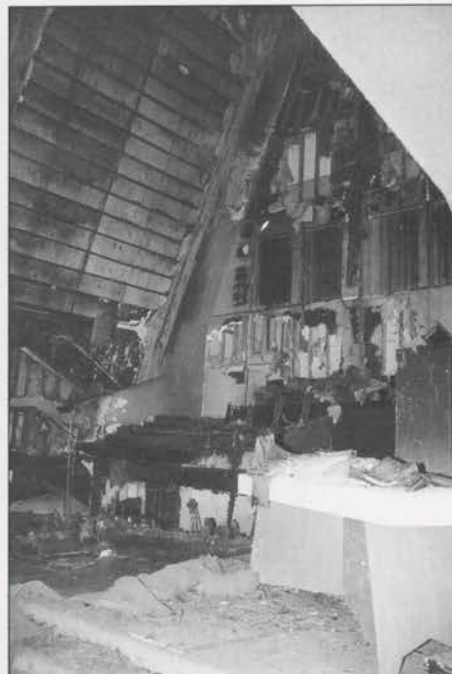
The sanctuary chancel. The fire was concentrated on the left side. The organ console fell through the burned chancel/choir loft floor and is a total loss. Holes in chamber walls are from firefighters looking for "hot spots."
