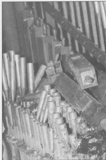
Tibia Clausa and Vox Humana pipes took a heavy blast of water from holes chopped in the walls.
