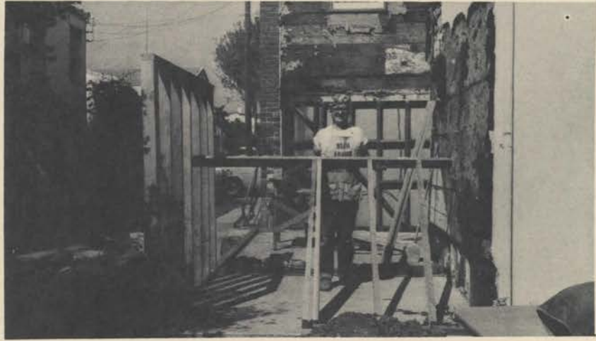
The author raising the 2nd section of framing on the newly poured floor slab, standing in the blower room - chamber at the rear.
