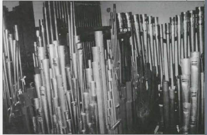
The Main chamber houses over 2100 pipes. Still, there is ample room for tuning and service work.
