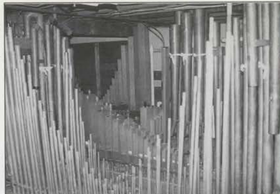
View of solo chamber in Bob Eyer, Jr.'s mostly-Möller home installation.
