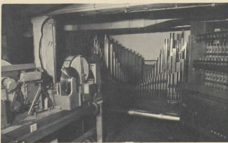
Toy counter on left, harp on right, with pipework in background, Joseph basement.
