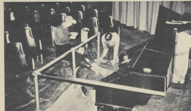
Kagy, Meier and Arey hard at it replacing flooring and installing protective rail around the console.
