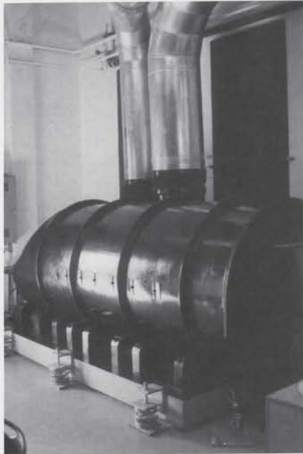
50 h.p. blower with spring shock mounts to eliminate vibration. Note steel strap plate for reducing or eliminating lateral movement in a major earthquake.
