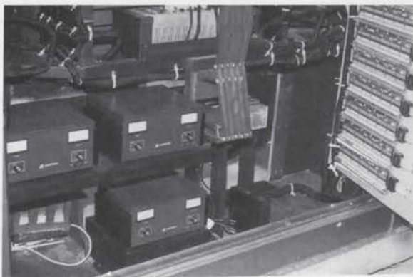
DC power supplies in console
