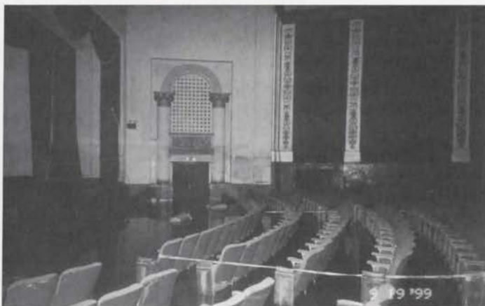
Saturday evening, the water still covered the front of the auditorium. The high water mark on the wall shows it came within 6" of the chamber
