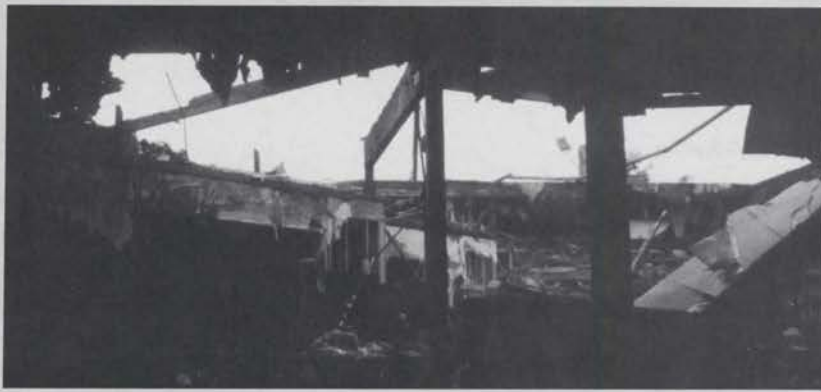
View to the outside through the collapsed roof.
