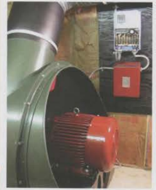
Blower room with variable frequency drive and load reactor cabinet.
