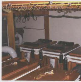
Overall quality of this installation depicted in restoration of main Chamber regulators.
