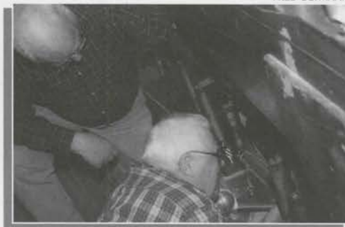
Joe Rementer (right) and Harold Ware work on the main windbox connection in the left pipe chamber of Cinnaminson High School.
