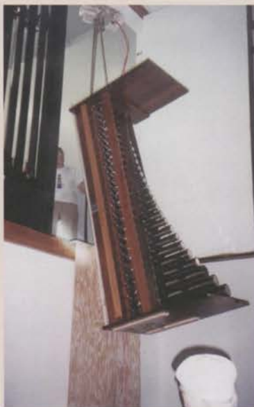
Large components, chestwork and blowers were moved into chambers before installing swell shades.
