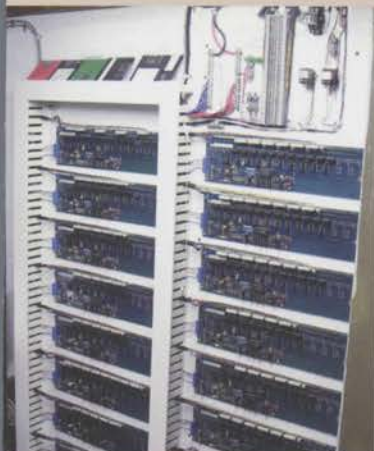
Z-tronics system racks.
