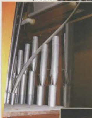
String pipe that "wilted" in the non-cooled theatre.
