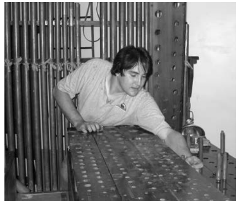
New York: Jesse Kohl installing rack boards on restored pipe chests at Long Island University (Photo by Tom Stehle)
