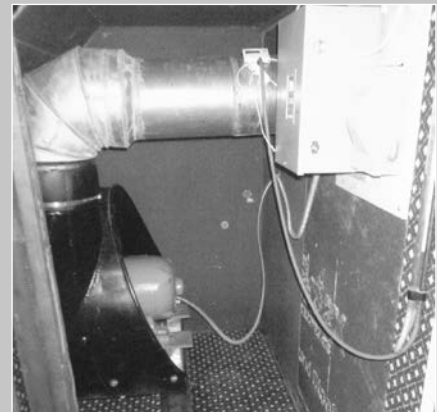
Blower room: 5-hp Spencer Orgoblo, powered by variable frequency drive
