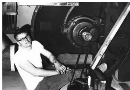
Ron and the 15 hp blower in the Albee basement, 1963
