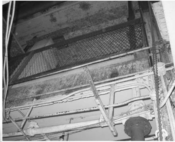
Note the chain link fence and railing in this photo. This is the mezzanine where such items as crated organ blowers awaited shipment
