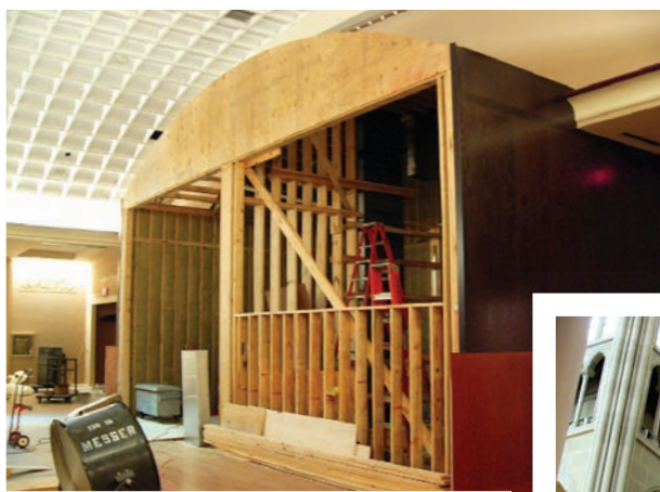
New chambers under construction in one end of the ballroom of Cincinnati Music Hall for the former Albee Wurlitzer (Photo by Robert Ridgeway)
