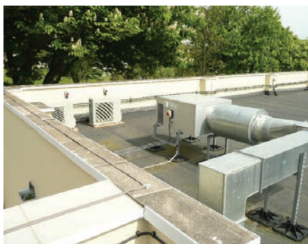
The critical air conditioning plant on the roof
