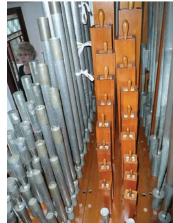
Pipes within the right-hand Solo Chamber
