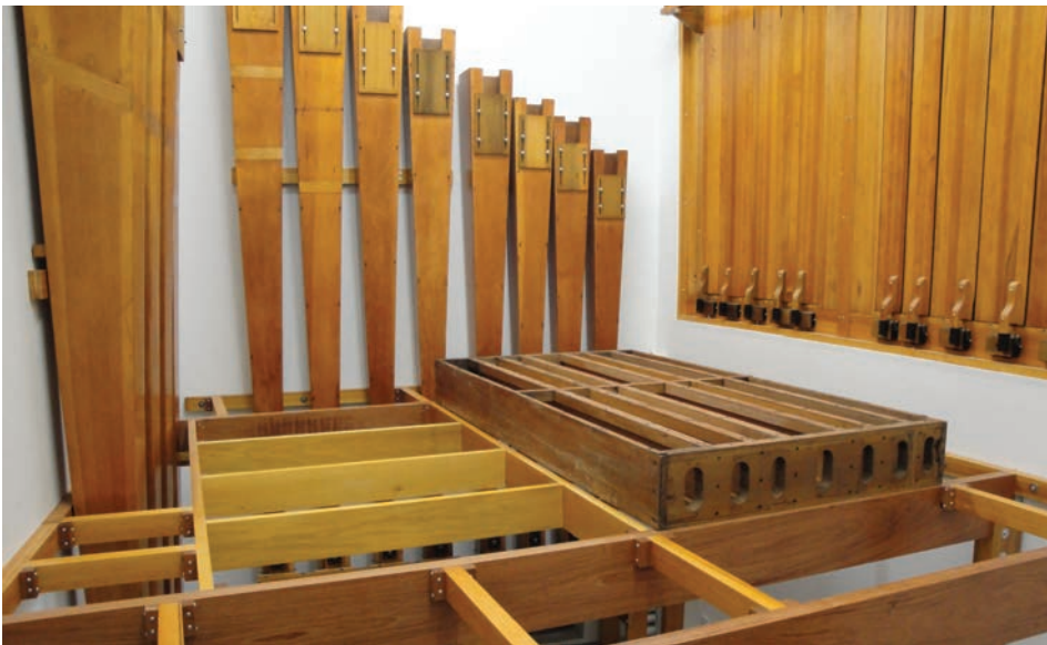
The short-span support pieces for the subfloor are Poplar; the ledger board circling the chamber is Robert-Morton (Photo by Bob MacNeur)
