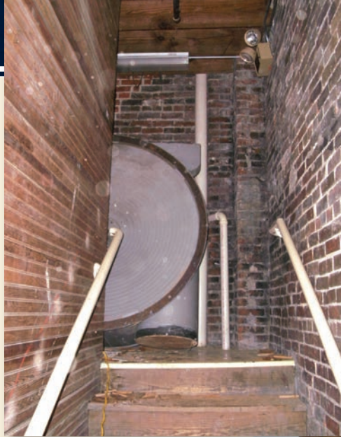
The blower tank had to be disassembled as much as possible to make the turns in the stairwell going to the blower room
