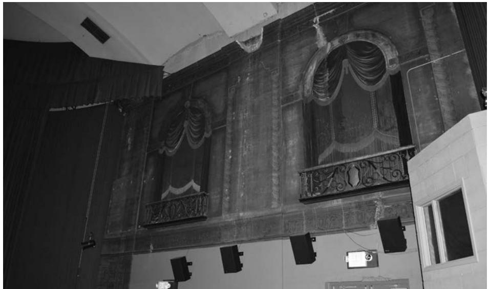
The "balcony" rails are metal; the rest is Trompe l'oeil. One of the old Cinerama projection booths can be seen on the right side of the picture
