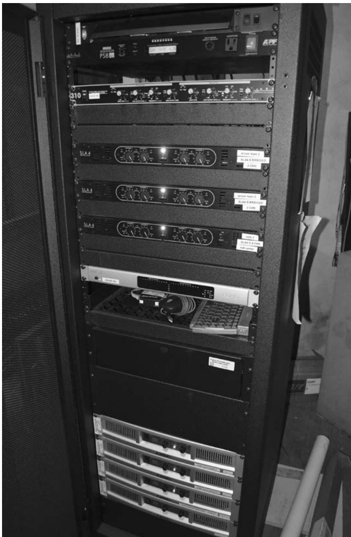
All the audio equipment is housed in a rack backstage, along with a power sequencer to bring on the amplifiers one at a time
