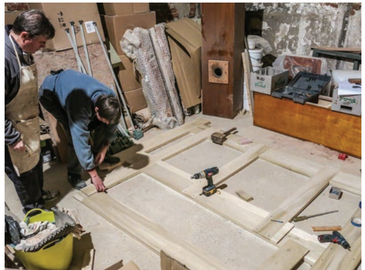
Building lower Main ground frame
