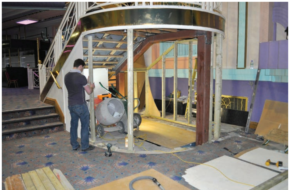
Console storage enclosure
