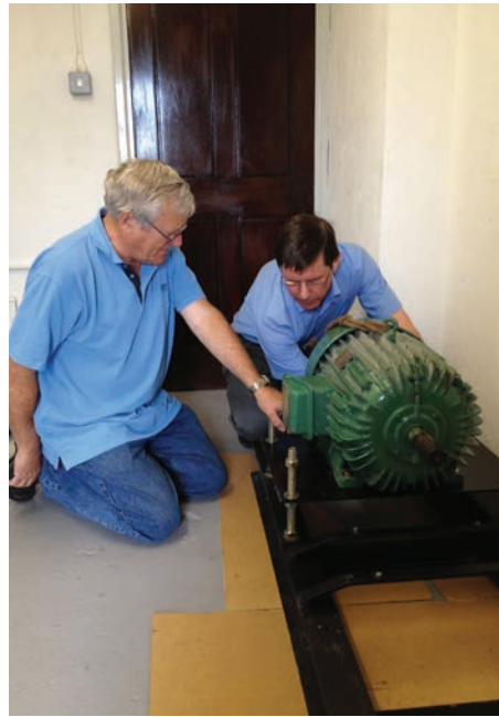
Main blower assembly
