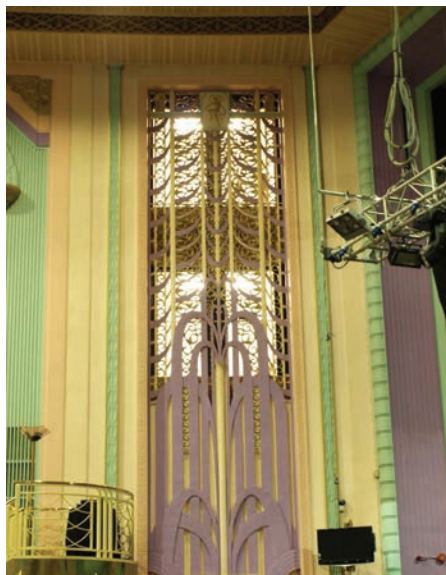
Main shutter frames
