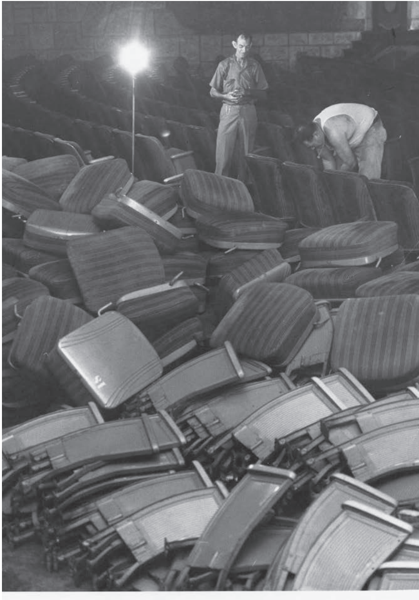
The Florida Theatre's Heywood-Wakefield seats being removed prior to demolition (Photo John Clark McCall, Jr. collection)
