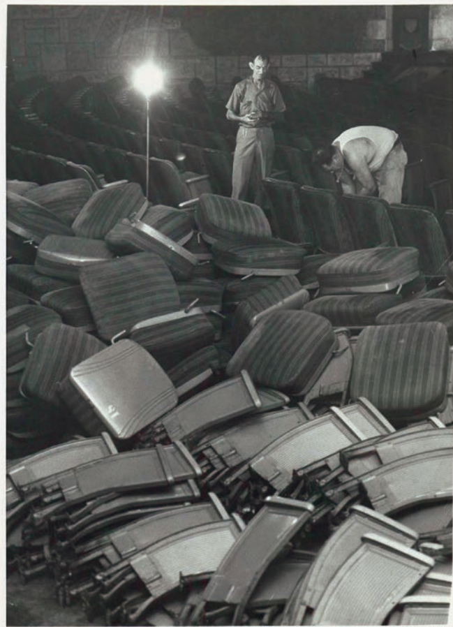
The Florida's Heywood-Wakefield seats being removed prior to the theatre's demolition. The Wurlitzer console can barely be seen in the upper right. The gentleman watching the workman is probably "Ash" Greeley, who was with the theatre from its opening day
