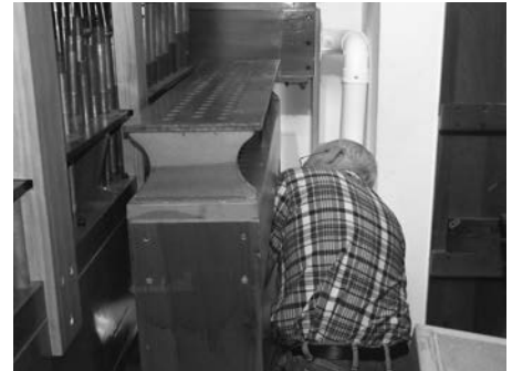
Ian Clark connecting the wind line to the Kinura chest (Photo by Ken Brown)
