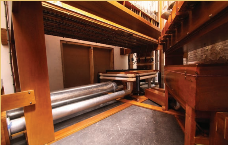
Beneath the Main manual chest, showing static windline, and large diameter regulated windline for offset chests. The unfinished wall section is a temporary panel. Eventually a removable panel will be put in its place to facilitate removing any large organ components in the future
