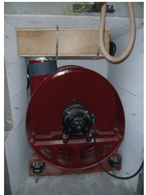
The blower in place in its vault; notice the wheels
