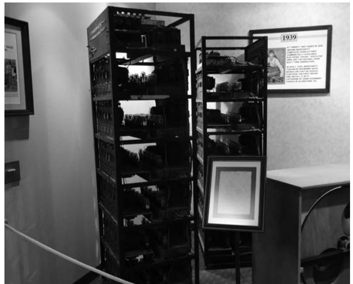
These are racks of tube-type tone generators from the early pre-transistor era.
