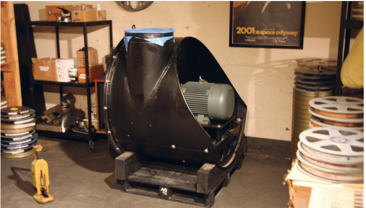
The blower is in place—it sits on a rubber pallet to decouple it from the floor and minimize rumble coming through the concrete
