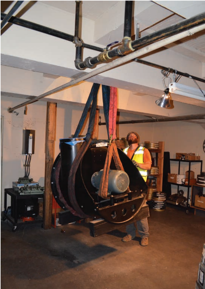
The blower had to be raised back up through the floor, and longer chains added. The blower wouldn't quite make it all the way to the floor of the basement otherwise.
