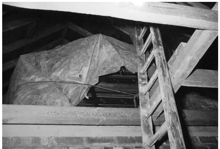
Removal of the relay from the Empire roof space (Len Rawle collection)
