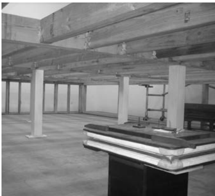
Space under chambers floor showing 2x8 joists and 6x6 floor support posts at Taylor building.
