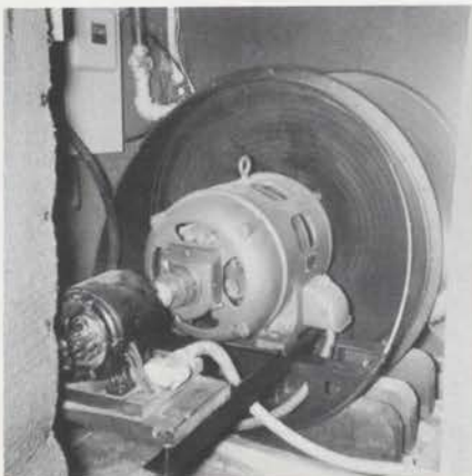
View of blower room with 10 horsepower single-phase motor showing the direct drive generator.
