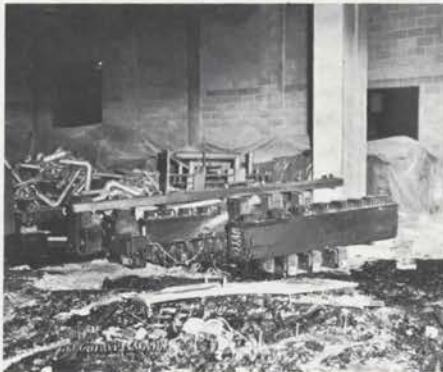
ANOTHER VIEW of damage, showing partially burned off-set chests, ashes of console again in foreground.
