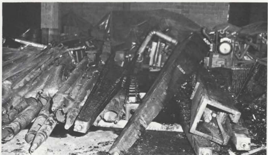
DAMAGED PIPEWORK clearly shows in this dramatic photo of a wanton attempt at purposeless destruction.
