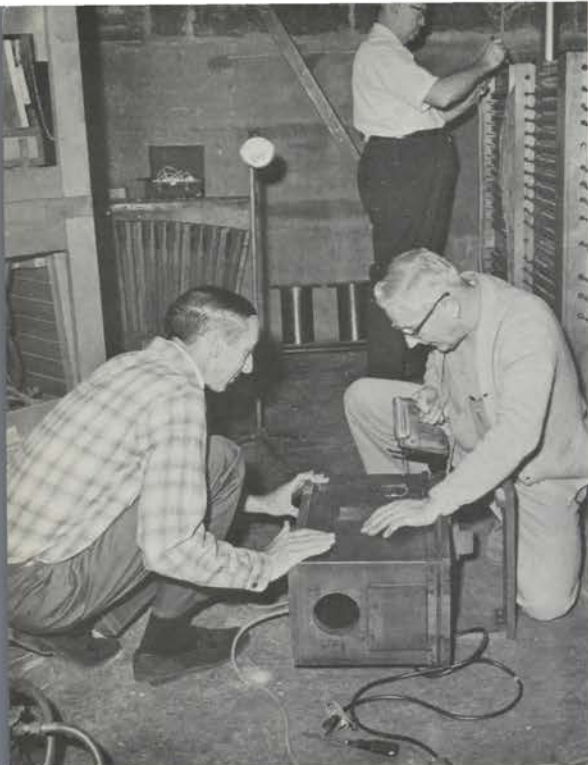
Bob St. John and Gil White operate on a static regulator while Hank Poole wires the relay.
