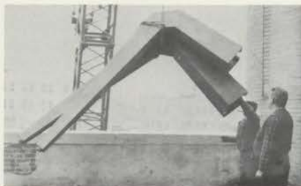
POP ART — A pair of enormous resonators forms an interesting composition as they are lifted from the roof of the Albee theatre in Brooklyn enroute to San Gabriel, California for reinstallation in that city's civic auditorium by members of the LA Chapter.
