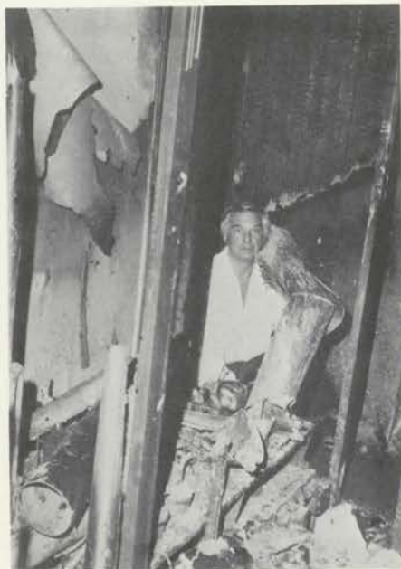
(Left) Solo Chamber. George among the remains of the 16' Tuba offset chest and melted Orchestral Oboe pipes.
