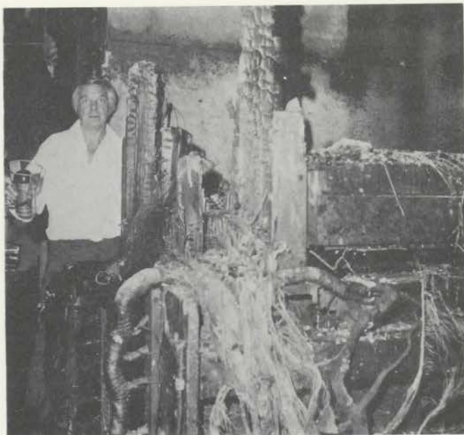
(Right) The charred relay room. George holds flashlight for photographer to focus.
