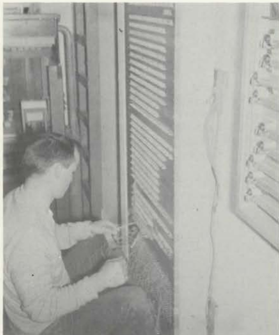
Otis Rashe solders final connections on junction board in relay room near end of 18 month installation period (1958-1960).
