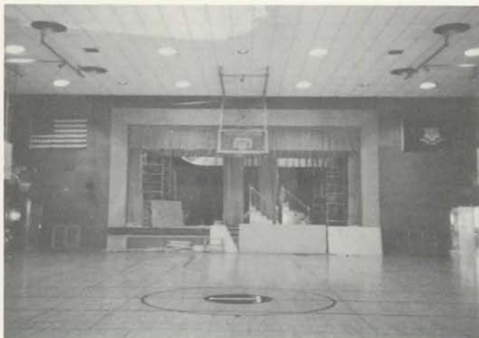
Combination Auditorium/Gym offers good acoustics. Piano, 16' wood diaphones and 16' Ophicleides will be placed against stage back wall. Chamber openings will be high on either side of stage where flags now hang. Chamber construction is evident from scaffolding erected on stage.
