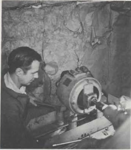
Leonard Worne tightens the mounting bolts on the low voltage generator after it has been coupled to the motor shaft — the final steps of the job. Note the acoustic material on the wall. This was done some time ago in an earlier attempt to reduce the noise conducted to the auditorium, but it didn't help much. The rebuild job did the trick.
