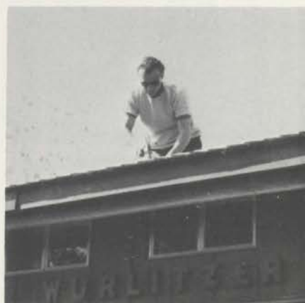
Son-in-law, Gerry Carver, putting the finishing touches on the roof of the Console Chalet.
