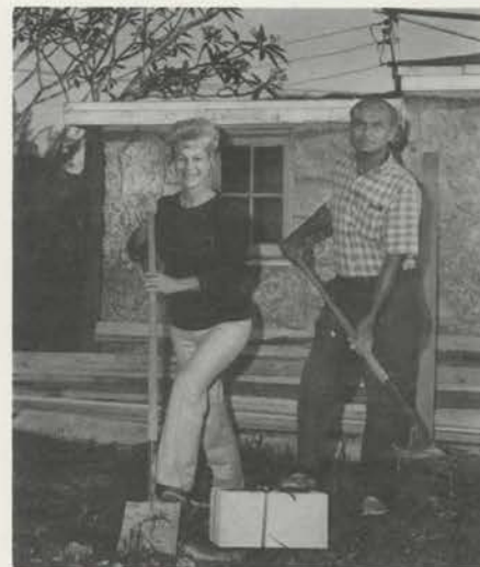
Chapter Chairman Bob Andre and wife Vivian break ground for new building to house Wurlitzer 260, formerly in Jacksonville's Florida Theatre.
