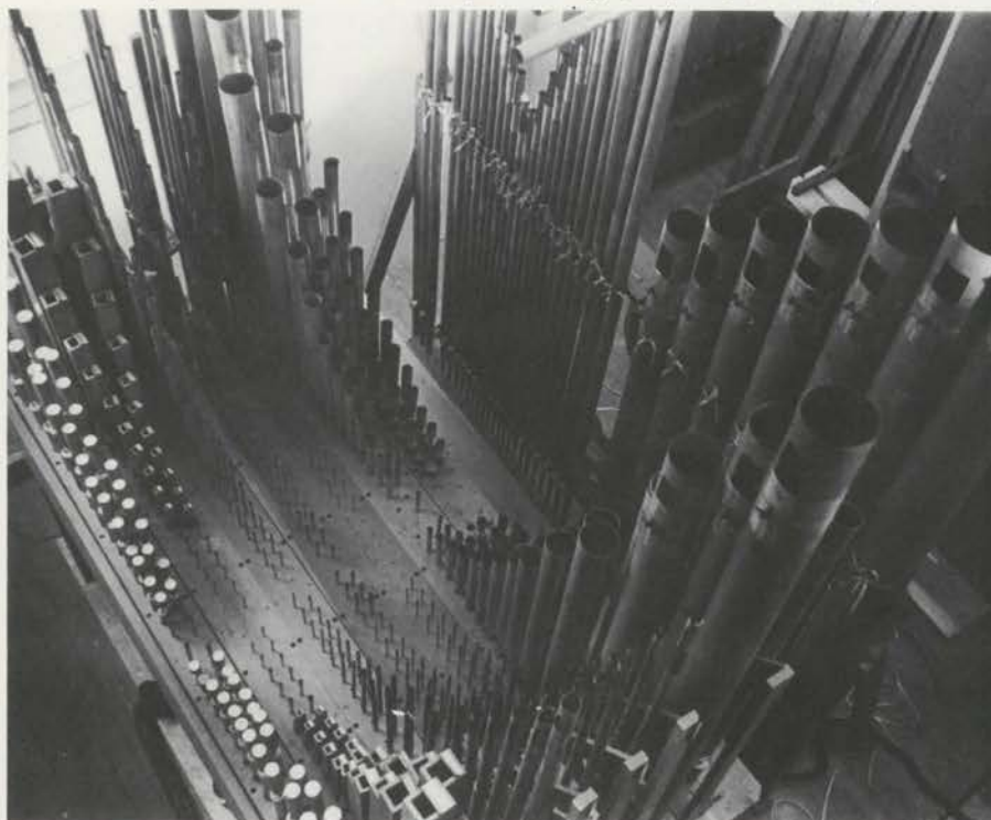
Pipe work in main chamber of CIPHER HILL organ. — (Dan O'Toole Photo)
