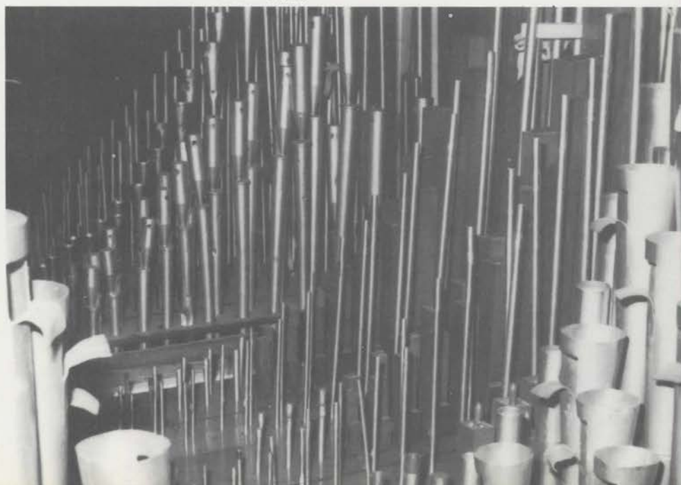
Main chamber of this unusual Wurlitzer organ.
