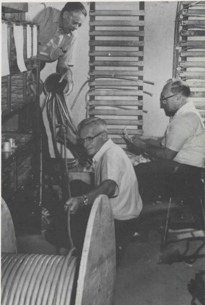
Standard 99-wire organ cable was used in underground ducts from blower room to relay room, above. George Allen leans over 2nd touch relay as Bob Lent separates wires for junction boards. Ed Dornfeld, foreground, at one time worked for Wurlitzer in the 40's.
