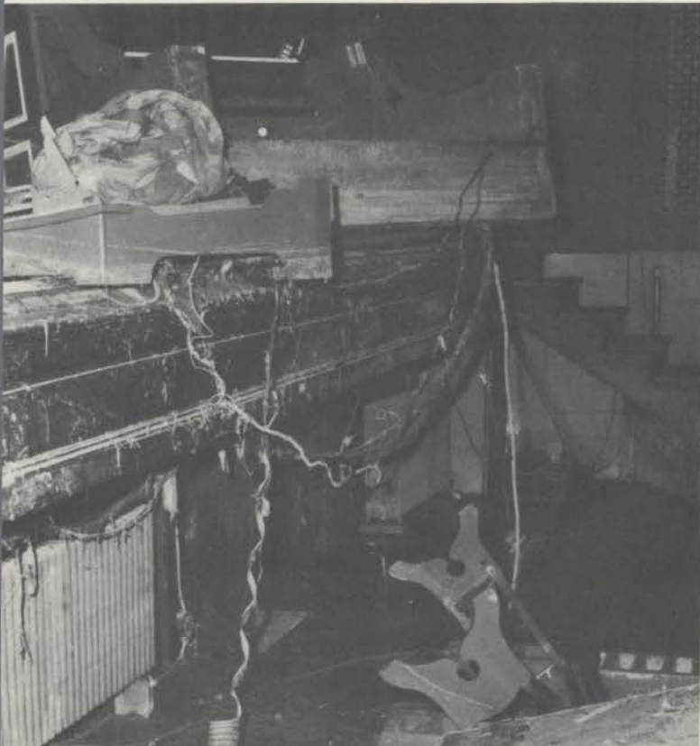
Tivoli Theatre orchestra pit after the floodwaters subsided. Console and pedal-board floated onto the stage.
