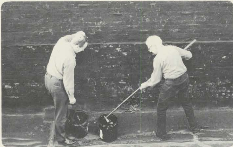
Bob Balfour (L) and Bob Reilly tar the roof of the Olde Rahway Theatre.
