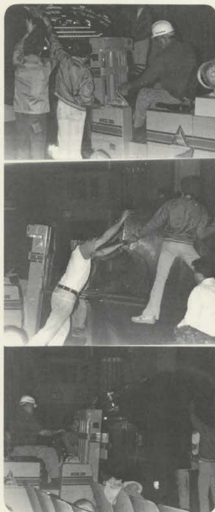
Red River members assist in placing the Fargo Theatre Wurlitzer on the new lift.
