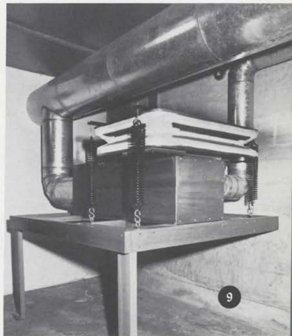
Regulator in basement for 16' extensions which are located on the stage. Large horizontal 14" windline is the main supply line for the Solo Chamber.
